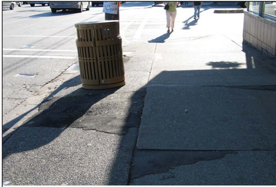
c) Sidewalk in Disrepair
